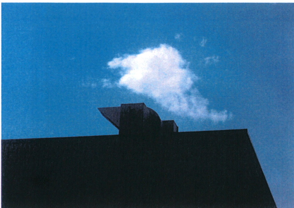
#3 - Headworks roof exhaust vent
