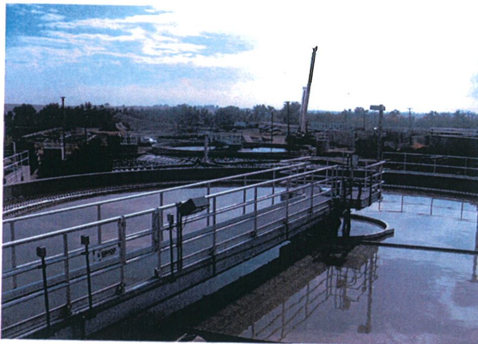
#12&14 - Primary clarifier (center)
