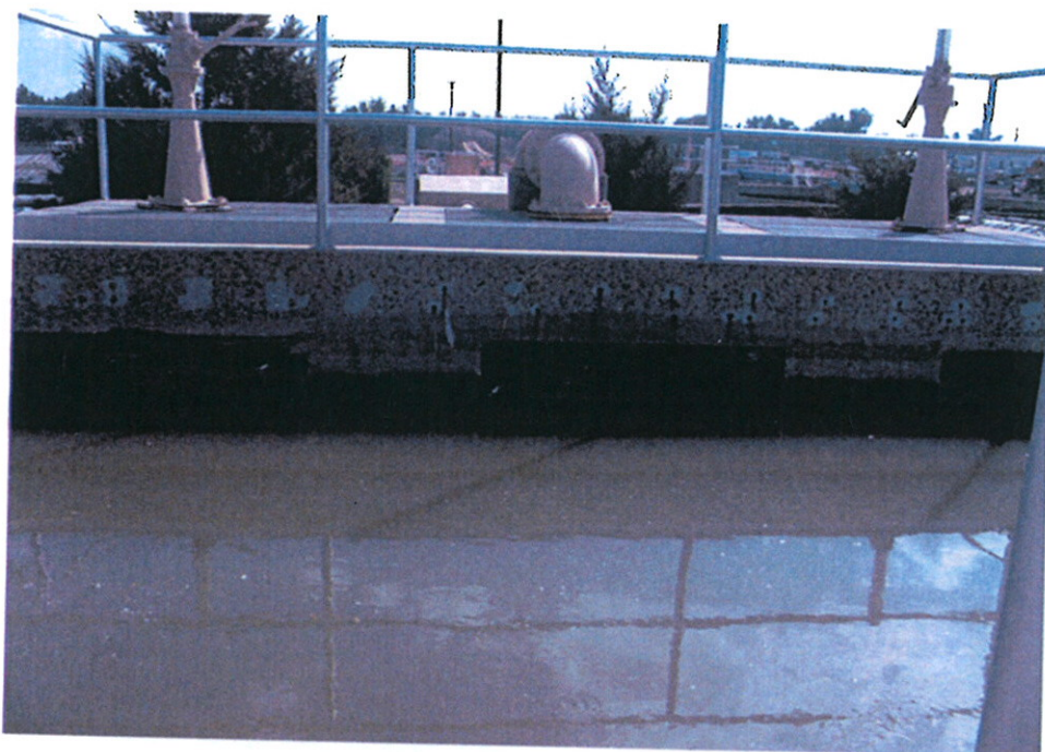
#16 - Primary effluent wetwell
