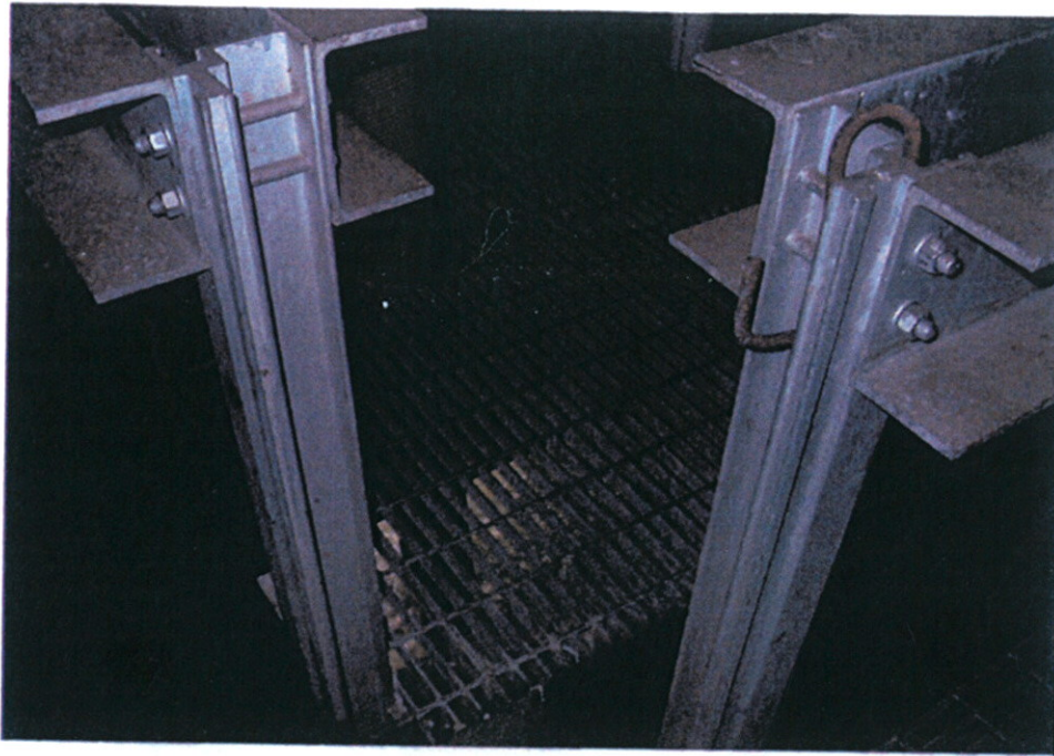
#6 - Headworks effluent junction box
