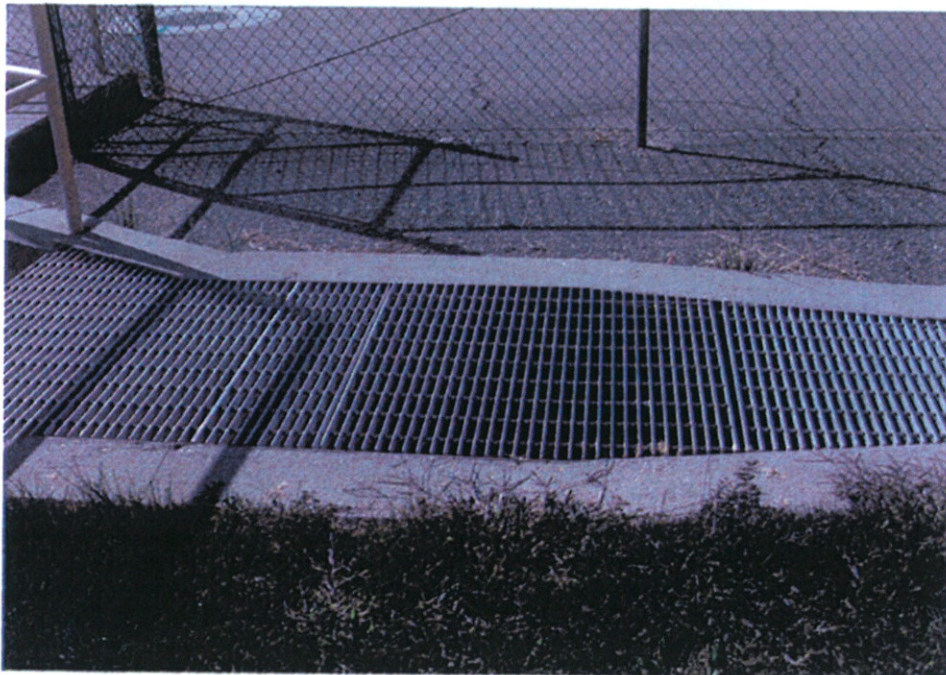
#8 - Aerated grit effluent channel (sample location)
