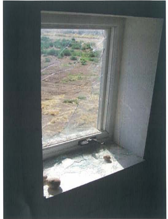
2007-HA-024 Milner Schwarz House September 21, 2007 Existing condition Image No. 149 Window Damage
