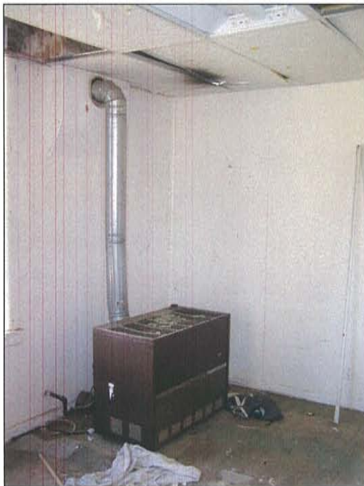
2007-HA-024 Existing condition Milner Schwarz House Image No. 092 September 21, 2007 Heater
