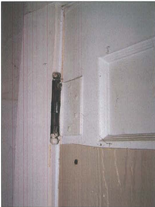
2007-HA-024 Milner Schwarz House September 21, 2007 Existing condition Image No. 134 Door Hinge Detail
