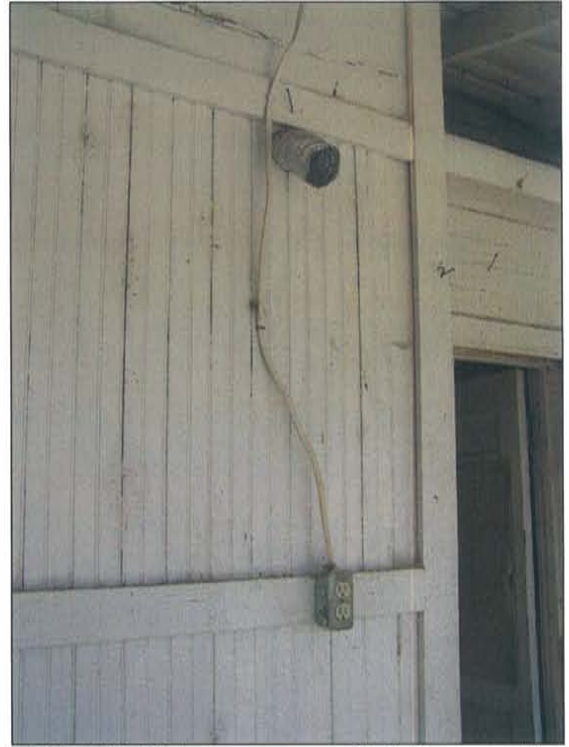
2007-HA-024 Existing condition Milner Schwarz House Image No. 031 September 21, 2007 Siding at Rear Porch
