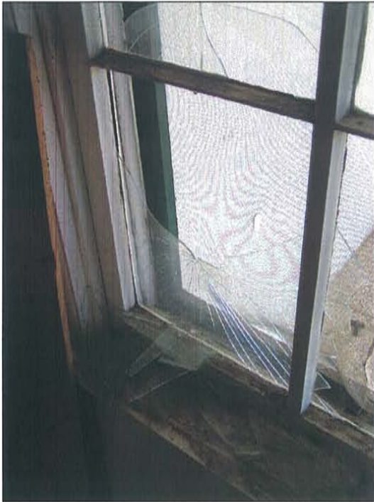
2007-HA-024 Milner Schwarz House September 21, 2007 Existing condition Image No. 148 Window Damage
