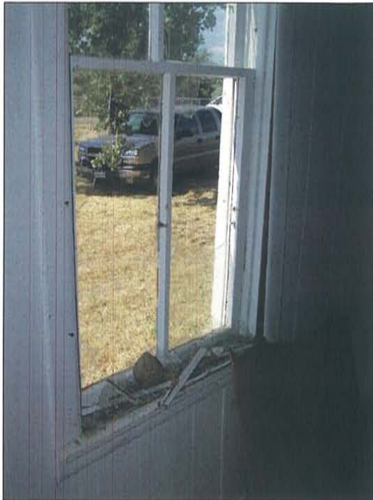
2007-HA-024 Milner Schwarz House September 21, 2007 Existing condition Image No. 152 Window Damage
