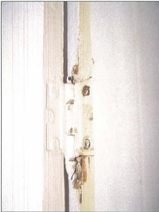
2007-HA-024 Milner Schwarz House September 21, 2007 Existing condition Image No. 141 Door Hinge Detail
