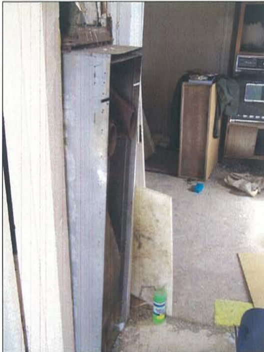
2007-HA-024 Existing condition Milner Schwarz House Image No. 090 September 21, 2007 Entry 101 Heater
