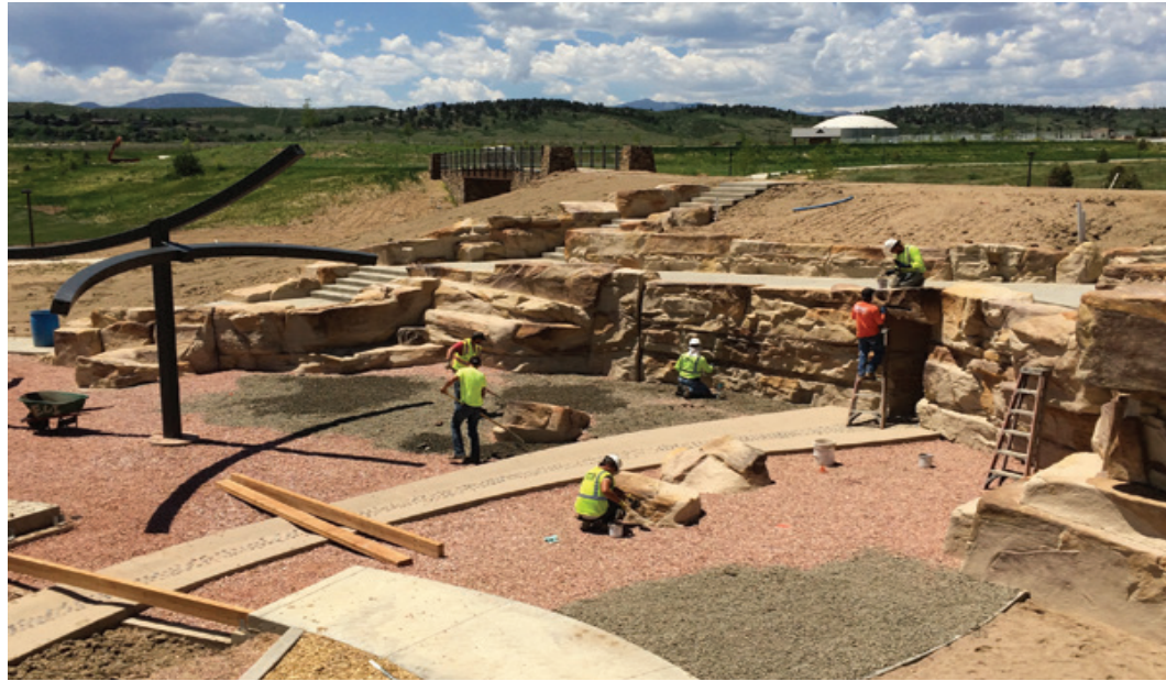
A small army of stone workers from Colorado Hardscapes Inc. swarmed over Mehaffey Park in mid-June, racing to get the play area ready for the new community park's grand opening.
