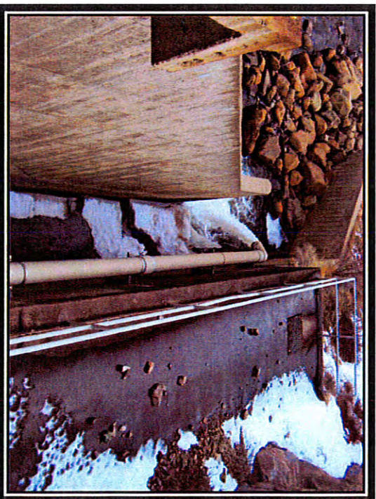
7.0 cfs minimum discharge low pipe, sluice gate channel, downstream view
